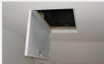
8: Clean out the plaster from between the door and the frame before emulsifying over ceiling and door face.
